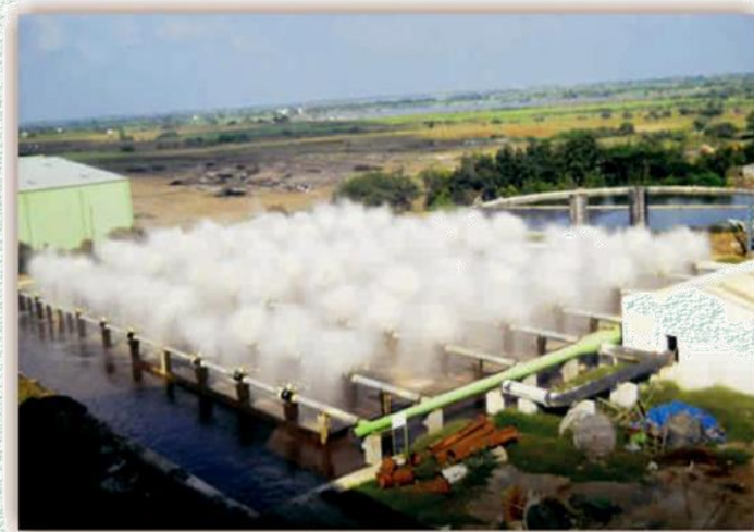
Advance Mist Cooling System.
